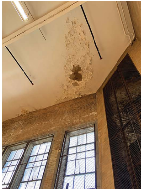
(b) Leaking Ceiling
