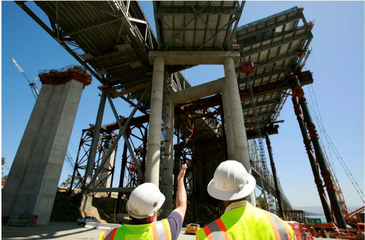
Reuters/ Robert Galbraith – A CalTrans worker displays a new section of roadway on the San Francisco Bay Bridge.
